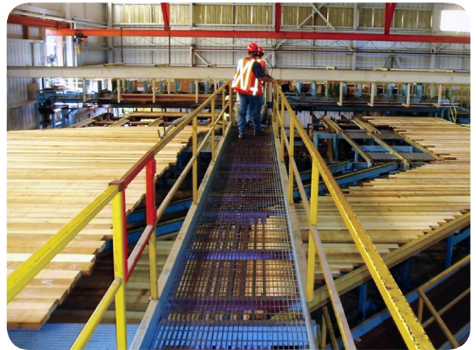
Work areas must be kept clear of wood dust buildups.
